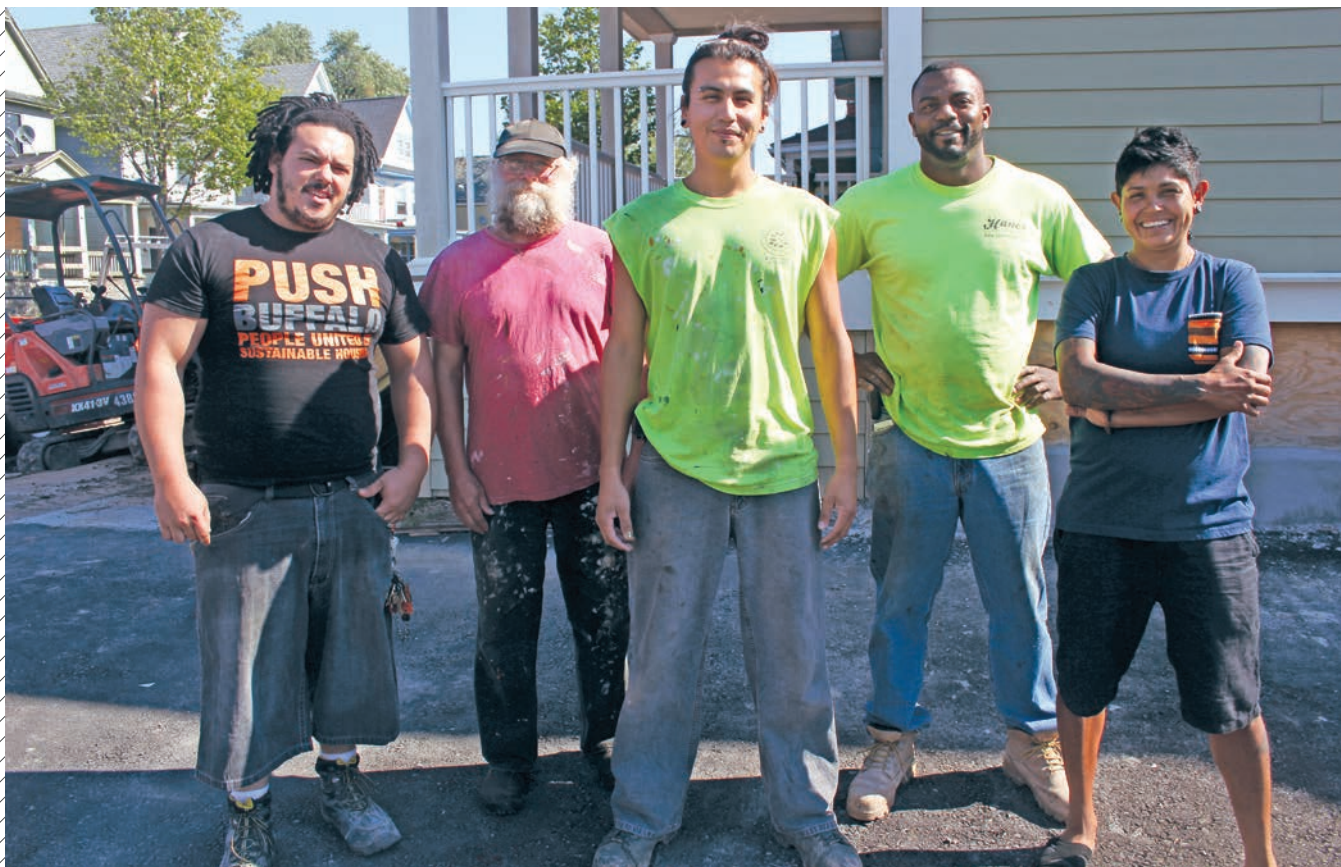
BELOW PUSH Buffalo’s Green Development Zone, which links the environmental movement to job creation, has received CFA support for sustainable development projects across Buffalo’s West Side. Below, the PUSH Buffalo crew excavates a site to support permeable landscaping and reduce impacts on Buffalo’s combined sewer system. Photo courtesy of PUSH Buffalo
