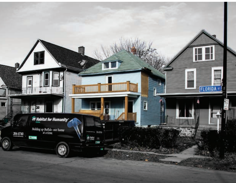
ABOVE: The renovation of 320 Florida Street, shown here during construction, will provide a family of Eritrean refugees with a home that can adapt to their needs over time. In supporting aging in place, the project also contributes to the stabilization of the neighborhood.
