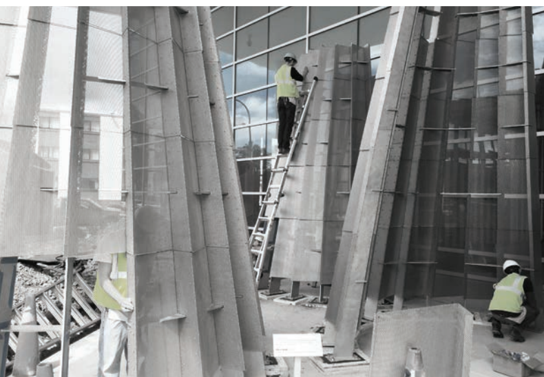
ABOVE: "Affine Shells" is a wind screen installation at the new Conventus building in downtown Buffalo. The conical forms of thin-gauge steel are the latest evolution of research by architecture faculty members Christopher Romano and Nicholas Bruscia with industry partner Rigidized Metals. Photo by Mahan Mehrvarz
