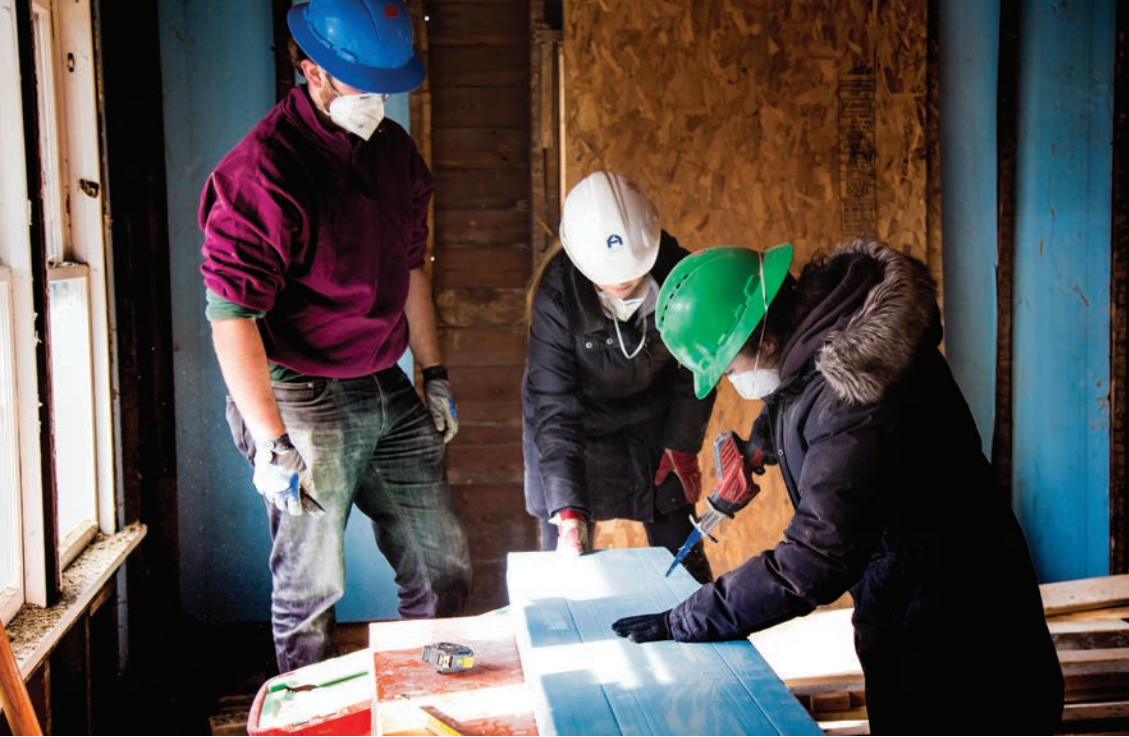
LEFT: The UB-Habitat Buffalo partnership, a core construction technology experience for hundreds of students over the past three decades, now includes a full design-build experience and opportunities to work hands-on with universal design. Photos by Alex Becker
